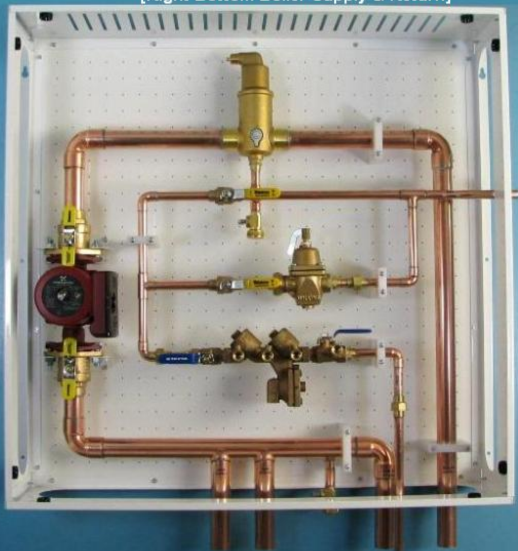
PLS-1RB [One Pump Primary Loop Station] [Right Bottom Boiler Supply & Return]
