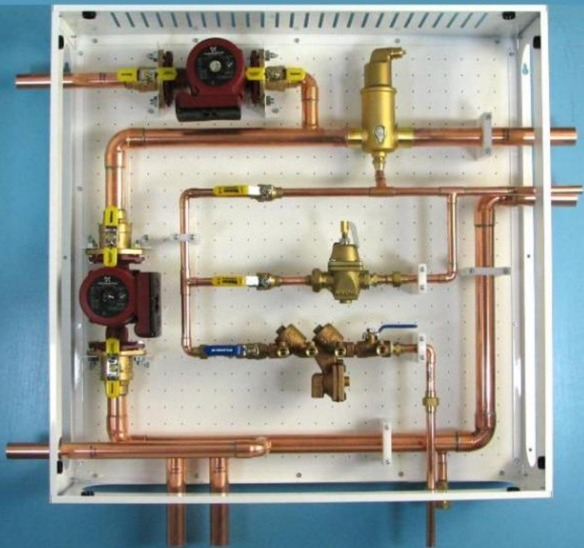
PLS-2RS Two Pump Primary Loop Station [Right Side Boiler Supply & Return]
